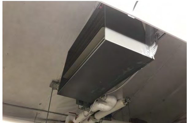
#22 UNIT HEATER IN MECHANICAL ATTIC
