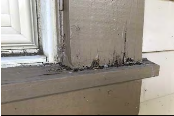
#13 WOOD ROT ON EXTERIOR WINDOW SILLS
