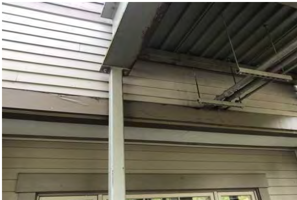
#11 WATER-DAMAGED WOOD TRIM
