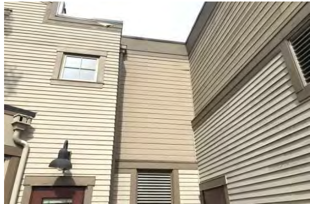
#10 WOOD SIDING DAMAGE
