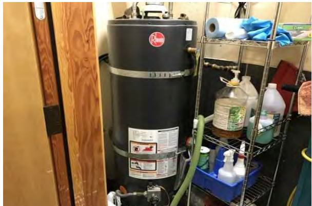
#30 DOMESTIC WATER HEATER
