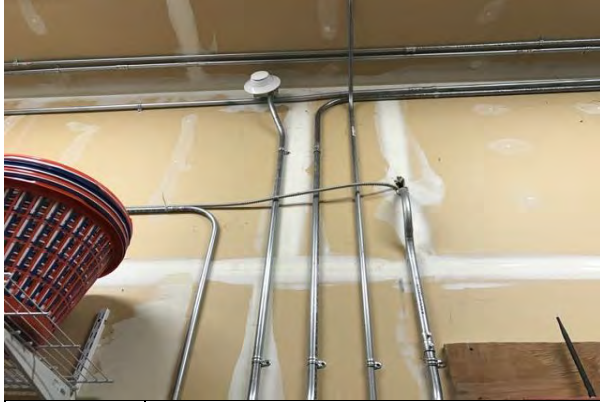
#43 NEW FIRE ALARM COMPONENTS
