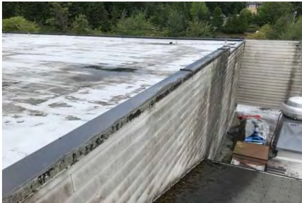
#9 FLAT ROOF DAMAGE AND GROWTH ON EXTERIOR WALL
