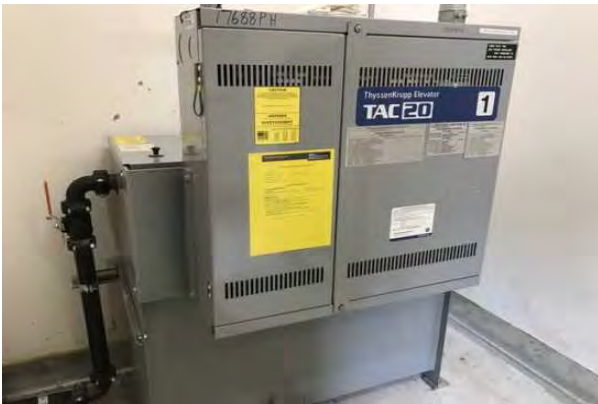
#17 HYDRAULIC ELEVATOR MACHINE
