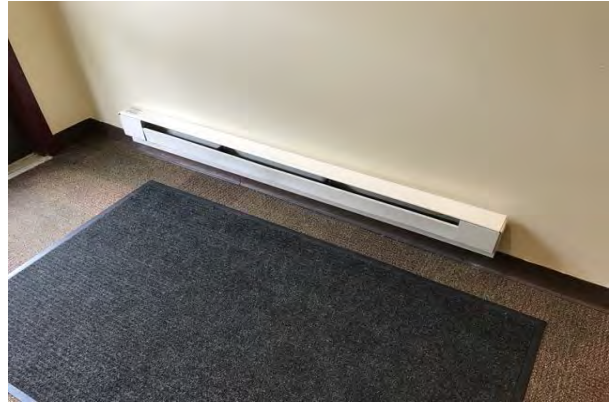
#38 HALLWAY ELECTRIC BASEBOARD HEATER
