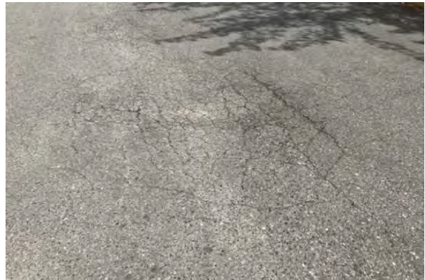
#46 ALLIGATOR CRACKING IN PARKING LOT
