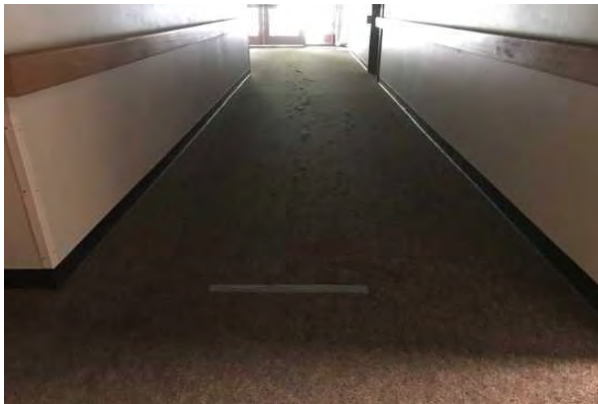
#11 DAMAGED CARPETING IN HALLWAY
