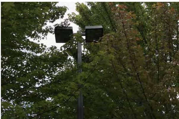
#30 EXTERIOR LED LIGHTING
