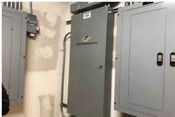
#29 PROBLEMATIC KAMELEON LIGHT CONTROLS
