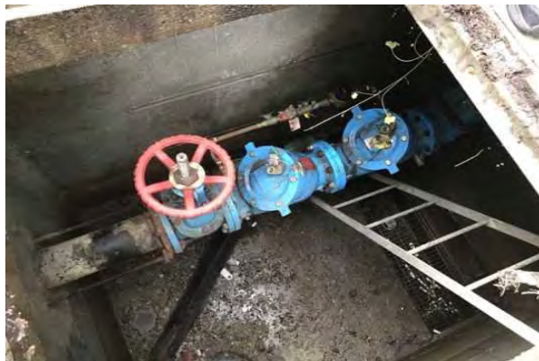
#39 FIRE PROTECTION BACKFLOW PREVENTER
