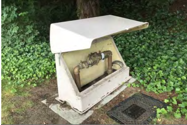
#31 DOMESTIC BACKFLOW PREVENTER
