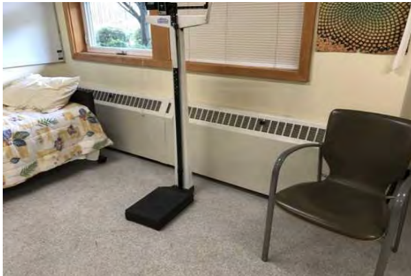
#21 HYDRONIC BASEBOARD HEATER
