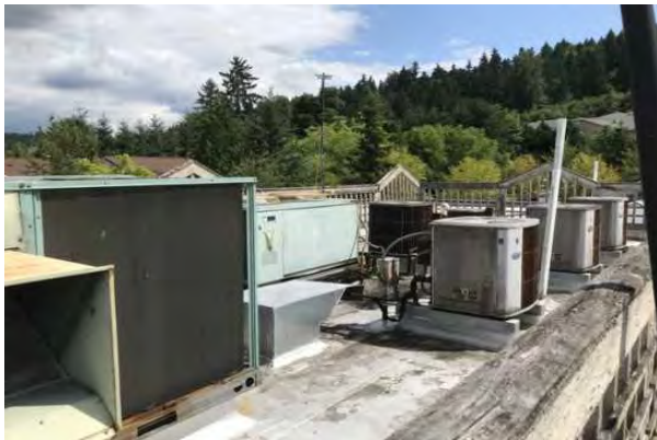
#35 ROOFTOP HVAC EQUIPMENT
