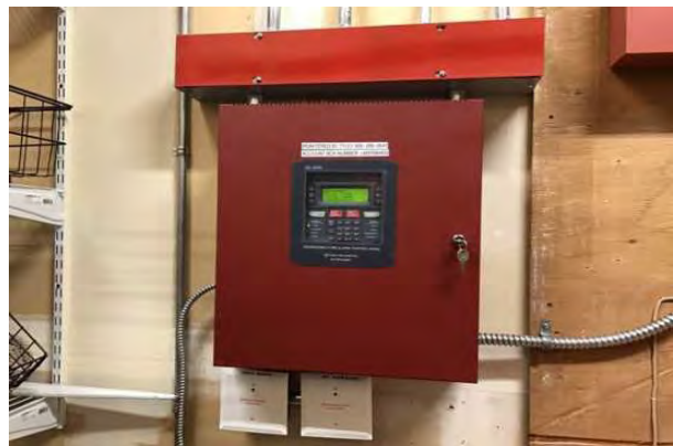
#42 FIRE ALARM CONTROL PANEL
