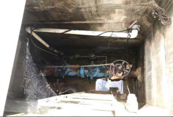
#26 FIRE SUPPRESSION BACKFLOW PREVENTER
