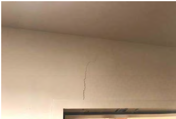
#5 SETTLEMENT CRACKING ABOVE DOORWAY
