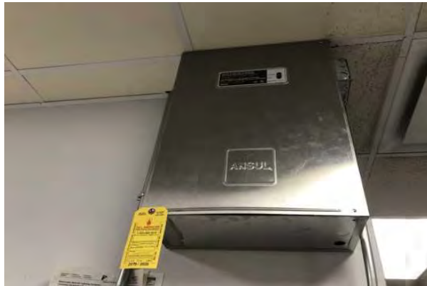
#27 KITCHEN SUPPRESSION SYSTEM
