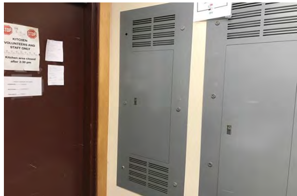
#40 ELECTRICAL PANELS IN KITCHEN
