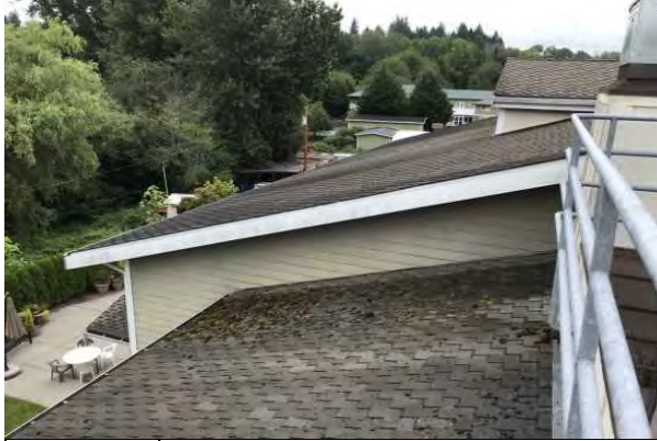
#7 ROOF VEGETATION GROWTH - REQUIRES CLEANING
