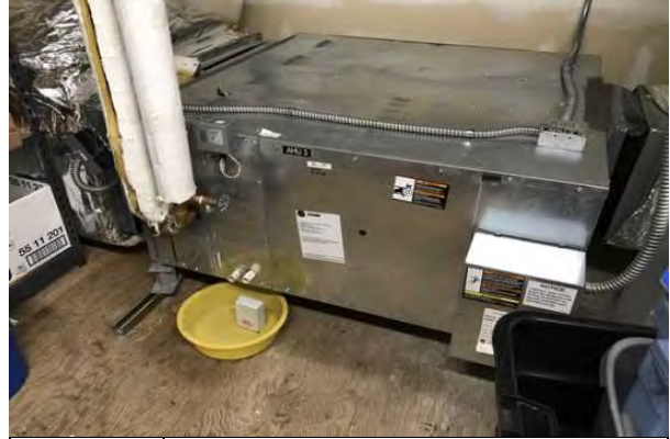
#20 INTERIOR AIR HANDLER
