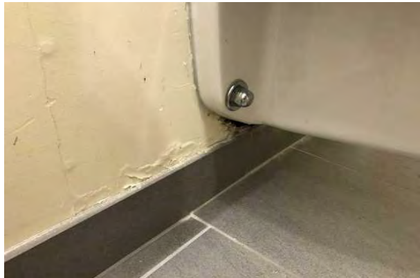
#34 PREVIOUS WATER DAMAGE - REQUIRES INTRUSIVE STUDY
