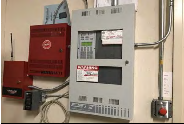
#31 FIRE ALARM CONTROL PANEL
