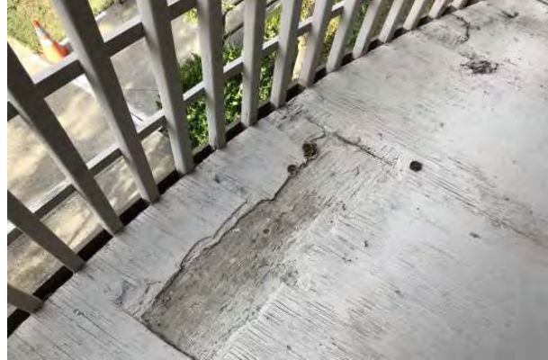
#8 DETERIORATING WOOD BALCONY STRUCTURE
