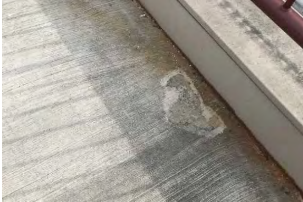
#7 CONCRETE SPALLING ON PEDESTRIAN BRIDGE
