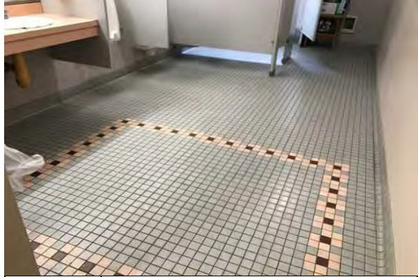
#32 RESTROOMS LACKING FLOOR DRAINS
