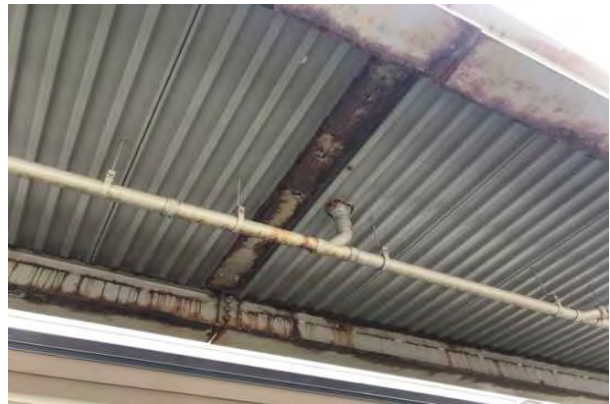
#6 SURFACE CORROSION ON PEDESTRIAN BRIDGE
