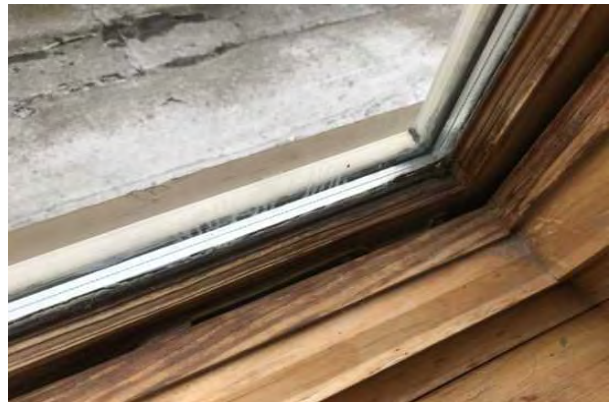
#12 INTERIOR WOOD WINDOW DAMAGE WITH WINDOW MOISTURE
